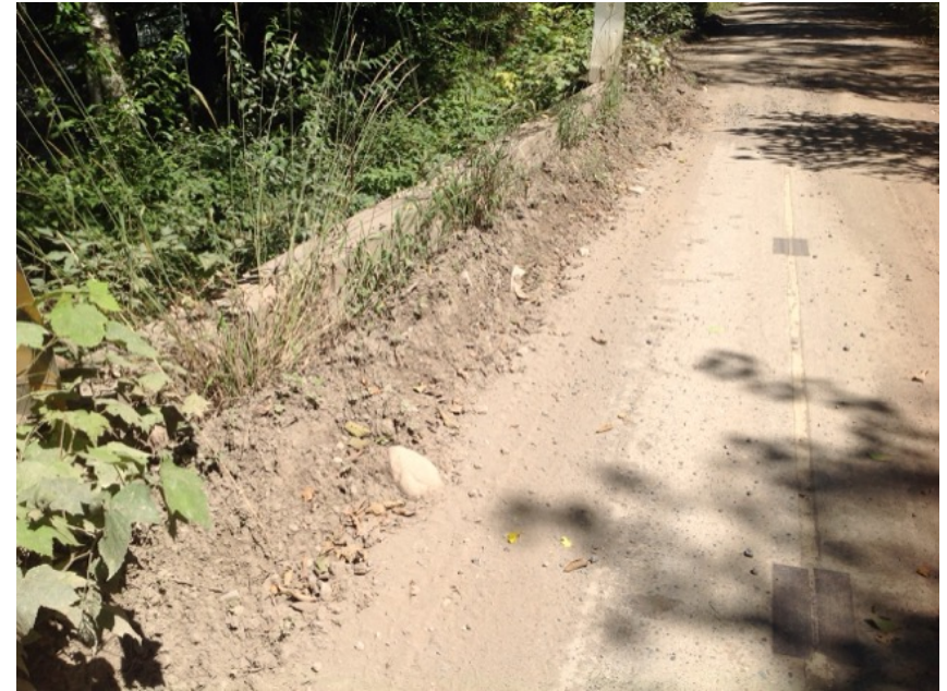
sediment accumulations against guardrail
